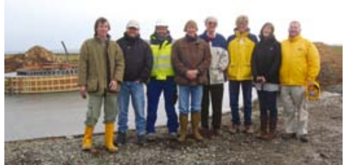
Building on success: The directors of TREL celebrate the completion of the foundations.
